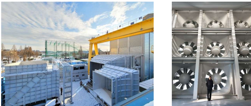
Figure 2. General view and 9(3×3) fans.
